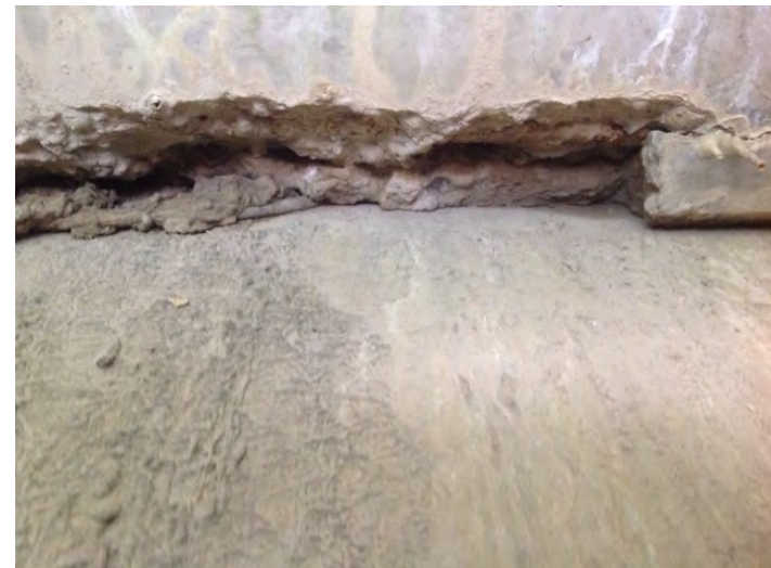
panel 1 damage underneath
